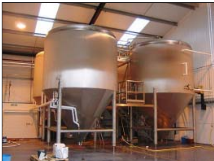
Equipment inside the new brewery
